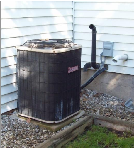
Air Conditioner Condenser Unit
