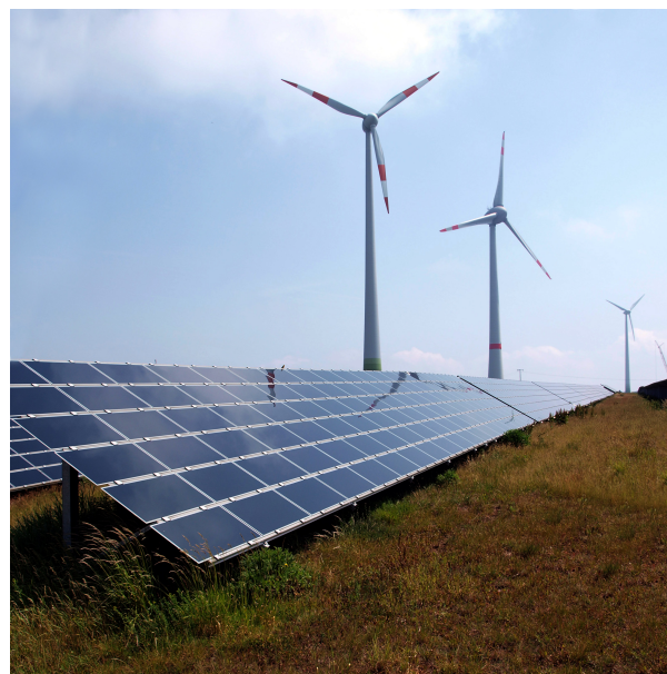
Figure 3: Photograph of Solar Panels and Wind Turbines.
