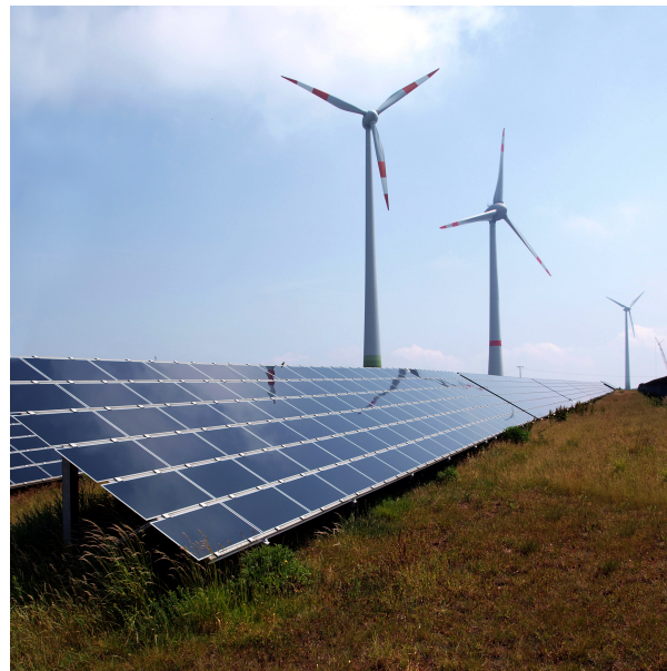
Figure 3: Photograph of Solar Panels and Wind Turbines.
