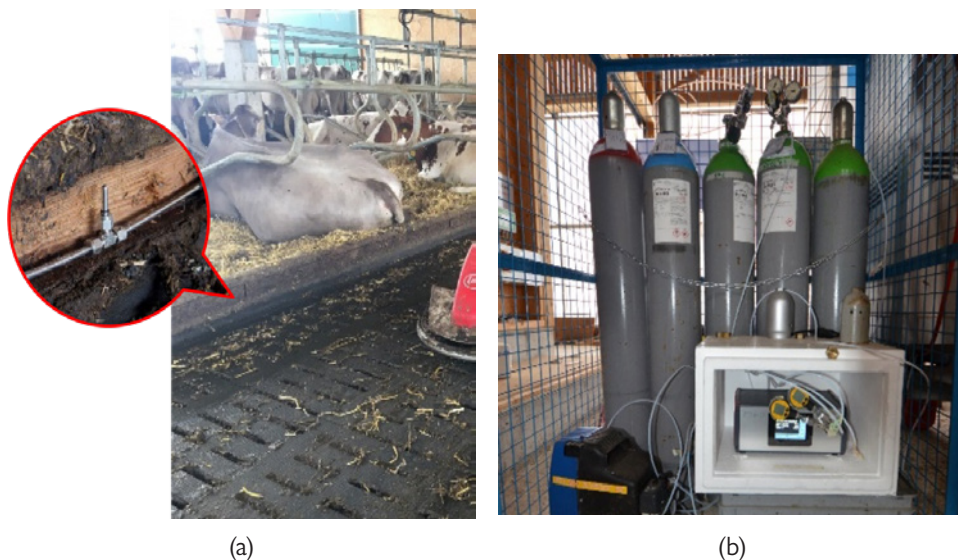
Figure 8. (a) Tracer-gas dosing by steel tubes with critical orifices protected by steel elements next to the floors in a dairy housing; (b) gas bottles with mass-flow controller.
