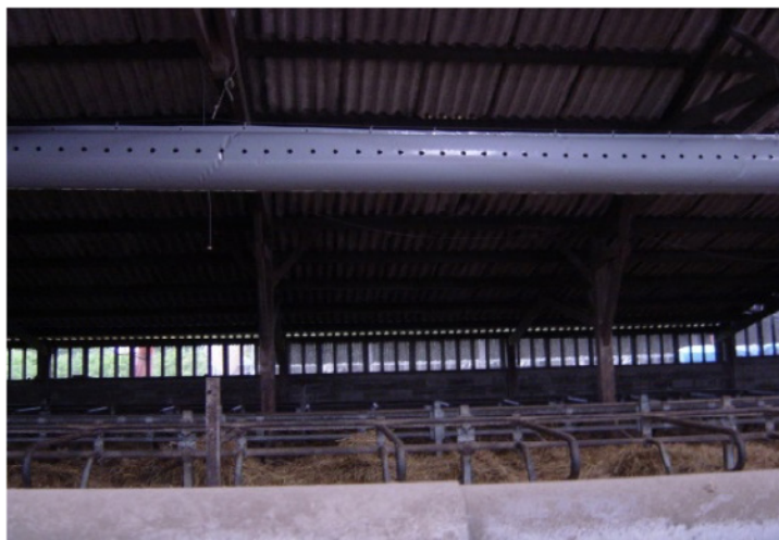
Figure 7. Duct for dispersing an artificial tracer gas within an animal house.
