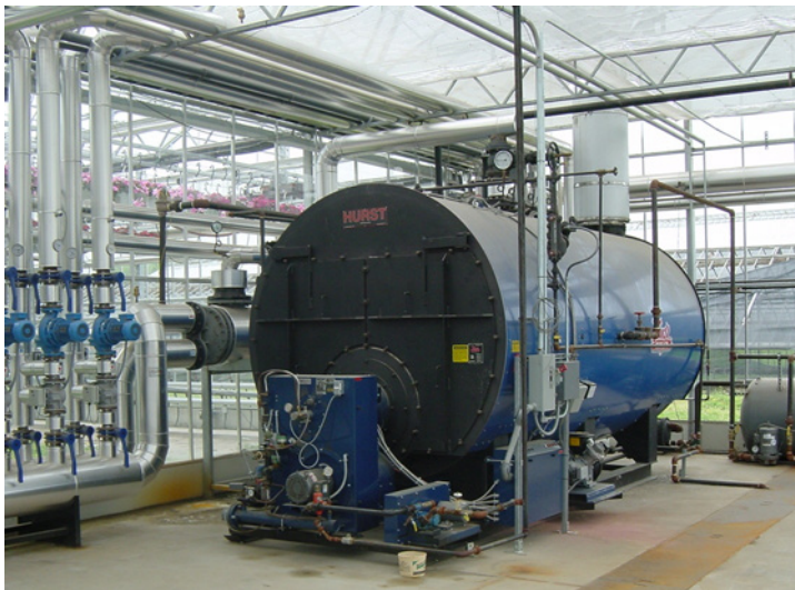
Figure 8. Hot water heating system including a boiler, mixing valves, pumps, and distribution plumbing (Photo by A. J. Both).
