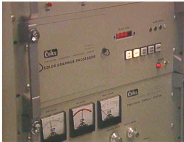
Celco 4000 Control Panel
