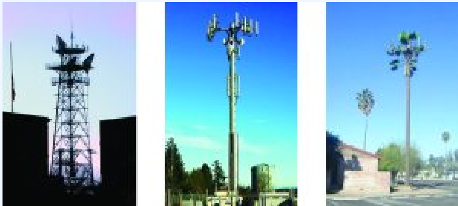
Figure 10.1d WIRELESS COMMUNICATION: Radio and cell towers are typically used to transmit long-wavelength electromagnetic radiation. Increasingly, cell towers are designed to blend in with the landscape, as with the Tucson, Arizona, cell tower (right) disguised as a palm tree. (credit left: modification of work by Sir Mildred Pierce , CC BY 2.0; credit middle: modification of work by M.O. Stevens , CC BY 3.0; credit right: work by Gary Minnaert , PD)
