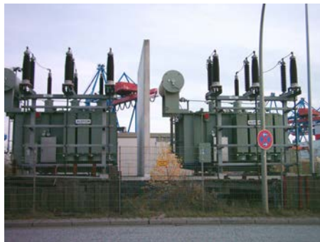
Figure 20.19 Power is distributed over large distances at high voltage to reduce power loss in the transmission lines. The voltages generated at the power plant are stepped up by passive devices called transformers (see Transformers ) to 330,000 volts (or more in some places worldwide). At the point of use, the transformers reduce the voltage transmitted for safe residential and commercial use. (Credit: GeorgHH, Wikimedia Commons)
