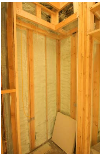
Figure 14.13 Insulation is used to limit the conduction of heat from the inside to the outside (in winters) and from the outside to the inside (in summers). (credit: Giles Douglas)
