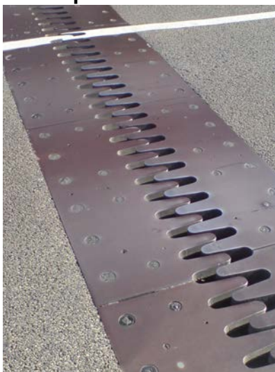
Figure 13.10 Thermal expansion joints like these in the Auckland Harbour Bridge in New Zealand allow bridges to change length without buckling. (credit: Ingolfson, Wikimedia Commons)
