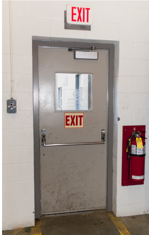
Figure 7 — Fire extinguisher near exit
