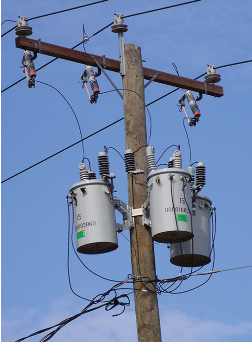
Figure 12.6.2 Transformers are used to step down the high voltages in transmission lines to the 110 to 220 V used in homes. (credit: modification of work by “Fortyseven”/Flickr)
