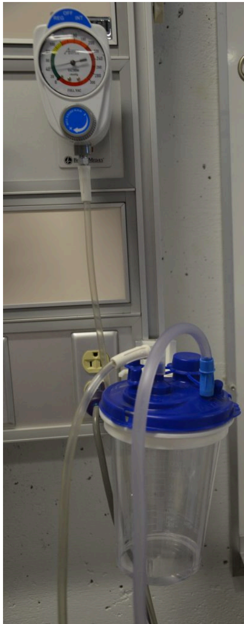
Figure 22.7 Tubing Attaching Suction Canister to Wall Suction Source
